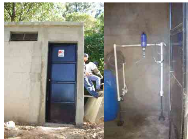
Water Quality Improvement Plan : Installed Sterilizer and the Shack
