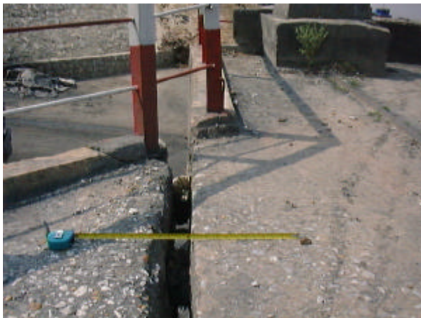
Gap between pier and access bridge
