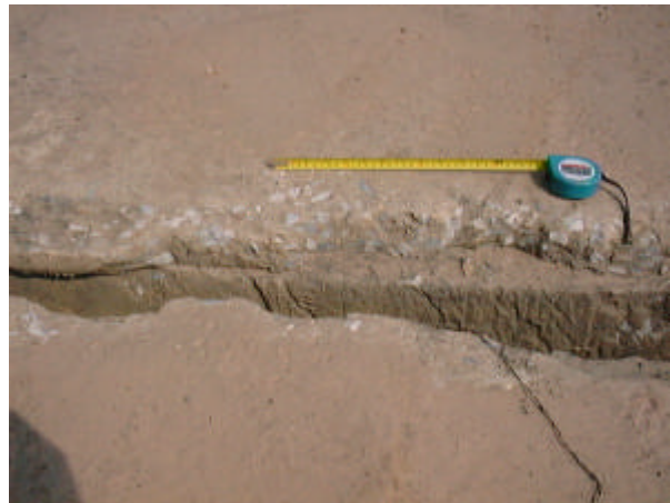
Crack and gap on upper slab between pier segments
