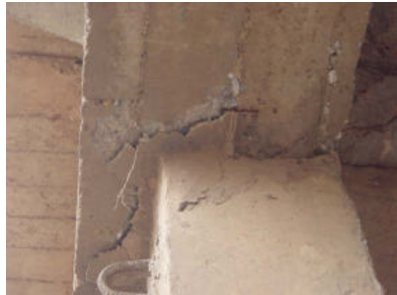
Damaged concrete pile due to excessive horizontal force
