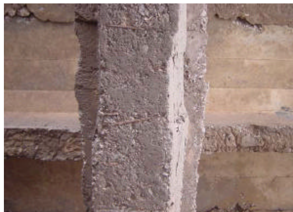
Deterioration of cross beam under slab
