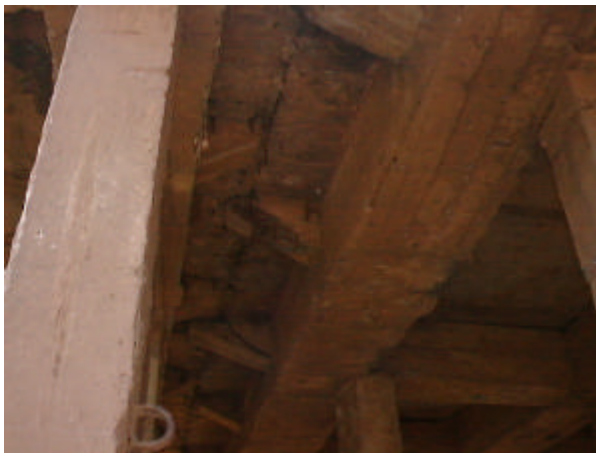
Crack and spalling of cantilever beam between pier and access bridge
