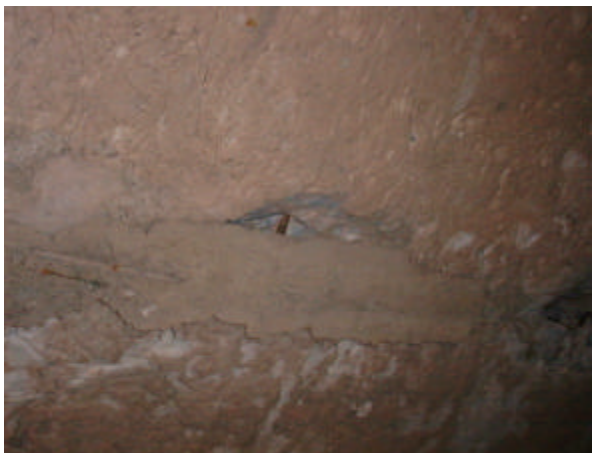
Damaged lower slab (spalling) due to thin covering and punching share
