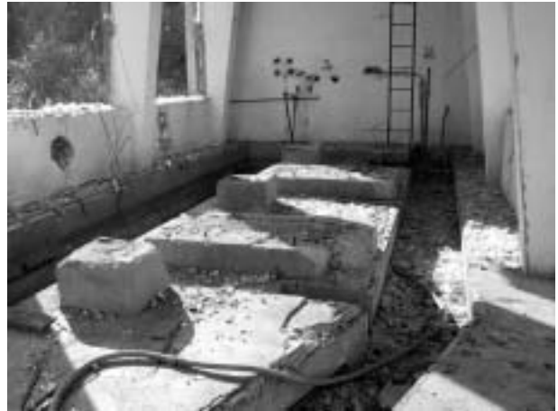
Remains of broken pump station. Pump was moved and windows were broken.
