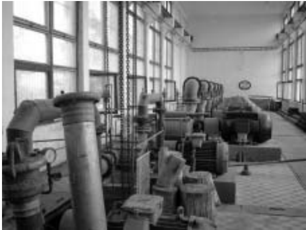
Dolecky Pump Station, Gajary (P.St-12)
