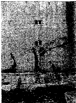
Connections between panels are not completed.
