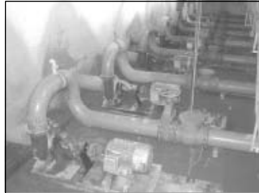
Scene of Inner Part of Tezeh-Abad Pump Station
