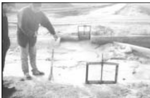
Silt Trap Condition in a Main Canal
