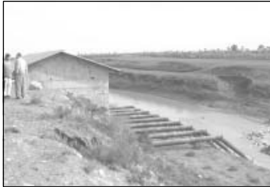
Scene of River Water Suction at Tezeh-Abad Pump Station
