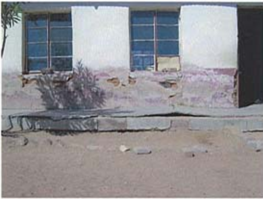
Deformity of structural slab and floated mortar
