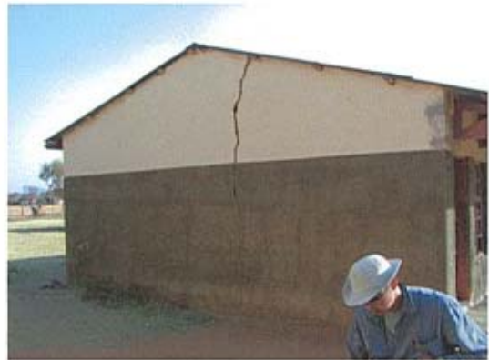
Structural crack on the gable wall
