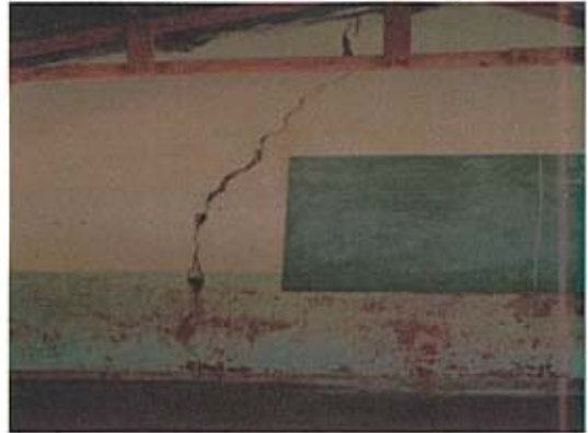
Structural crack on the front wall of classroom
