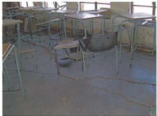
Structural crack at slab on earth by settlement
