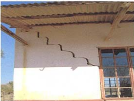
Another type of structural crack on the upper wall
