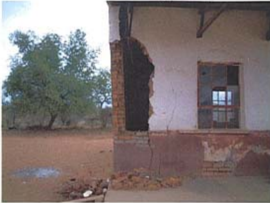
Breakdown of a corner wall and inclination of gable wall
