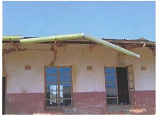
Structural crack at the upper part of window openings
