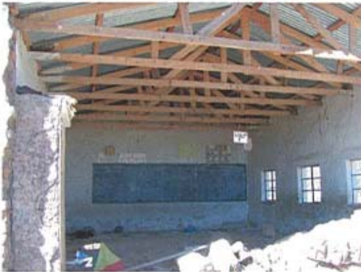
Complete collapse of the gable wall by foundation defect
