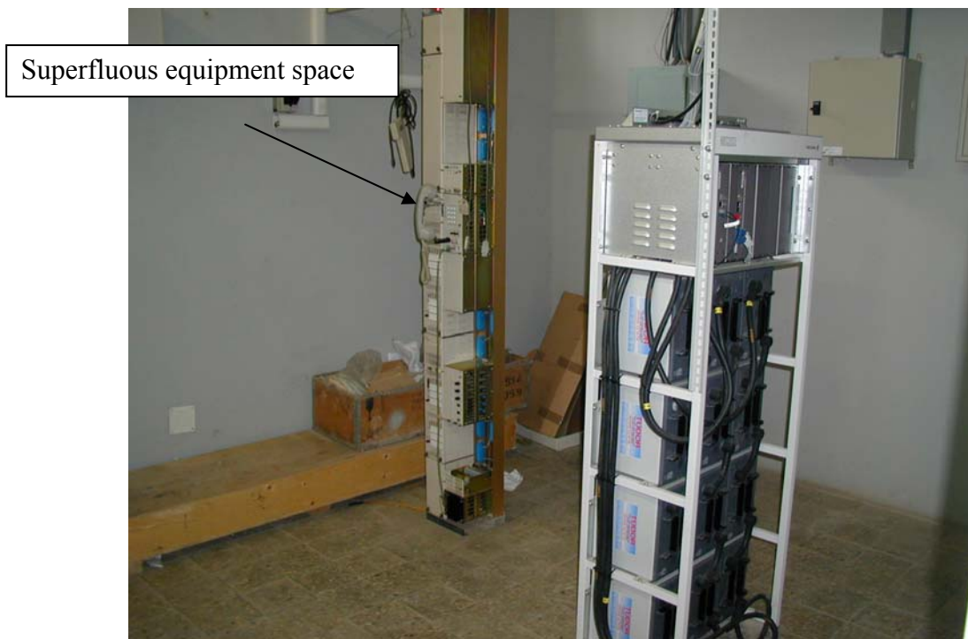
Photo No.15 : Superfluous Equipment Space in the Second Equipment Room in Debre Zeit
