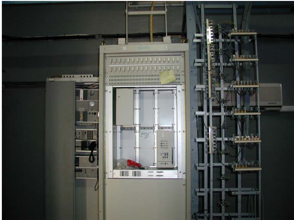
Photo No.16: The Idle Equipment (Siemens bay) in Adama West Rep., Which need to be moved in Advance.
