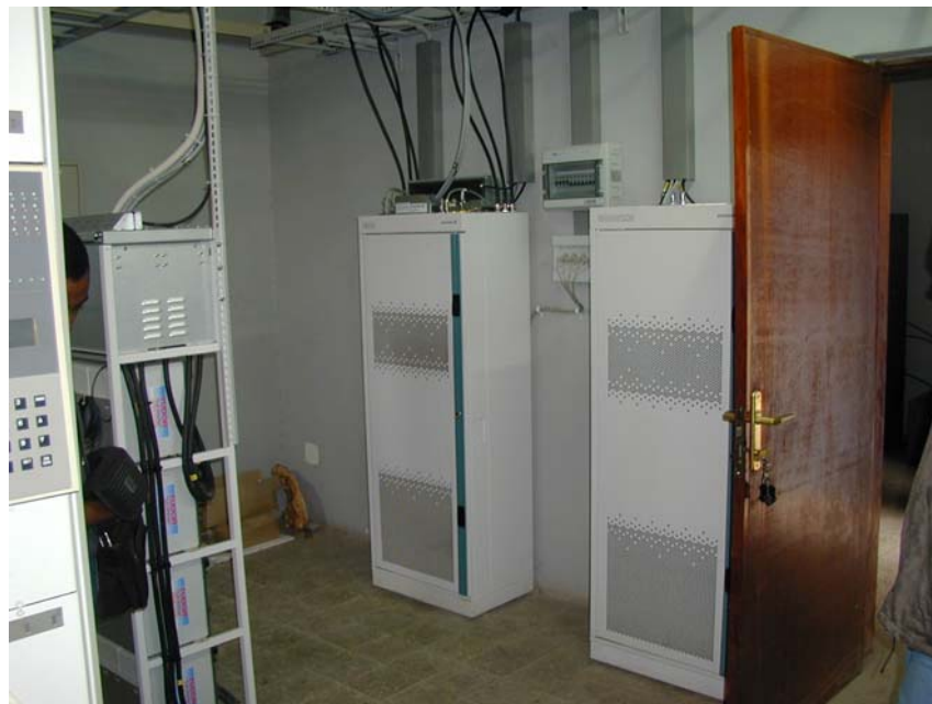
Photo No.9 : Expansion Space of the Existing Radio & Transmission Multiplex Equipment Room in Debre Zeit Telecommunications Second Station Building
