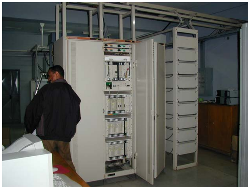
Photo No.13 : The Existing Radio & Transmission Multiplex Equipment Room of the Nazareth Primary Center
