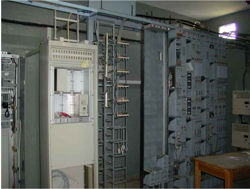
Photo No.11 : The Existing Radio & Transmission Multiplex Equipment Room in the Adama West Micro Wave Repeater Station
