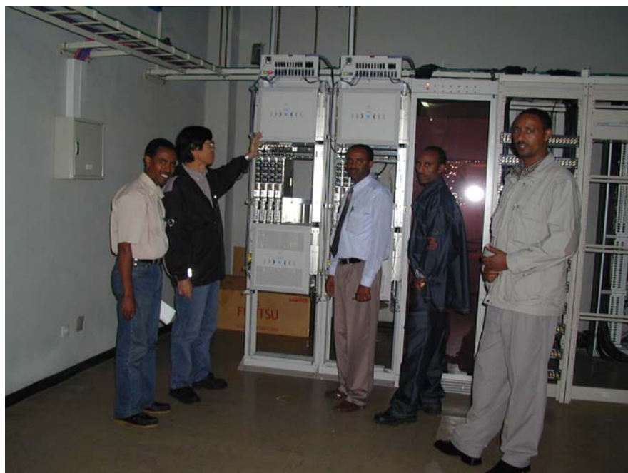
Photo No.7 : The radio & Transmission Multiplex Equipment Room in Addis Ababa-NEFAS Silk Telecommunications Center Building. As Survey, F/S Team verified Enough Free Space.
