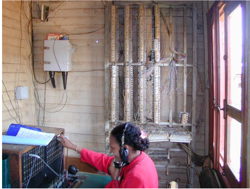
Attachment – 6 Operator telephone Booth (Manual Switching) in ETC Woreta Tele-house (DRMASS subscriber lines for manual switching assigned three lines (3CH))
