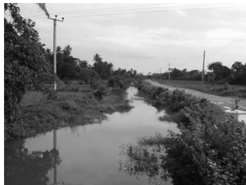
5-23 View of middle reaches of Maha Ela Photo was shot from Horana Road Culvert to downstream.
