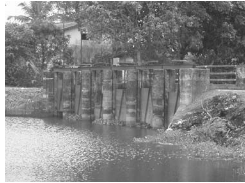
5-11 View of existing gates at Attidiya Irrigation Department office Photo was shot from right bank in upstream.
