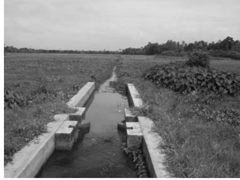
5-22 View of middle reaches of Depawa Ela Photo was shot from Egodawatta Mawatha Culvert to downstream.
