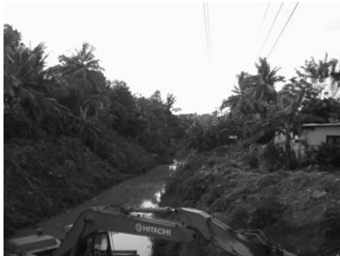
5-9 View of upper reaches of Bolgoda Canal in Dehiwala Channel improvement work of lowering channel bed by 0 m MSL was proceeded.
