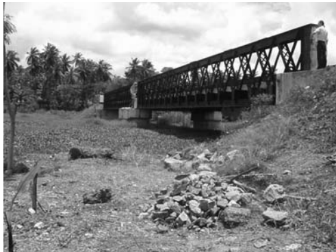
5-2 Upstream view of Borupana Bridge Steel girder bridge with two spans of 30 m
