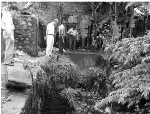
3-3 View of Inlet of Existing Mutwal Tunnel Photo was shot from upstream side.
