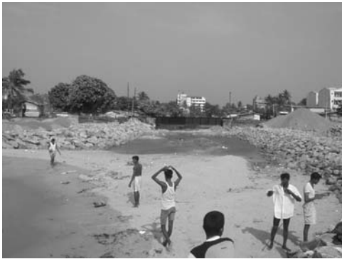
3-2 View of construction of jetty at outfall of Dehiwala Canal Photo was shot from sea side in March, 2002
