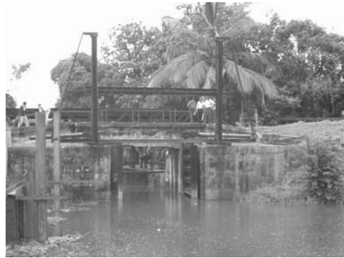
3-5 View of Existing North Lock Gate. Photo was shot from inland side. North Lock pumping station was studied in this location as an alternative measure.
