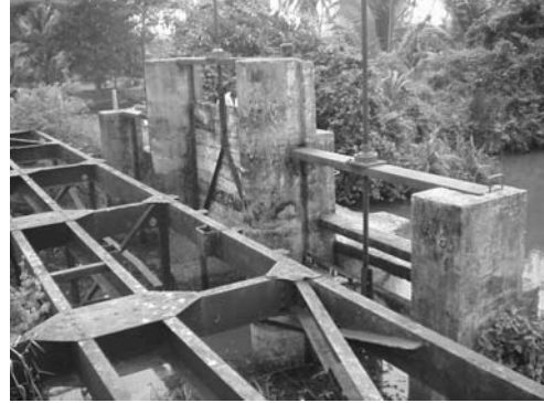
1-10 Southward view of Old Negombo Canal Gate Gate is installed at the confluence with Dandugam Oya
