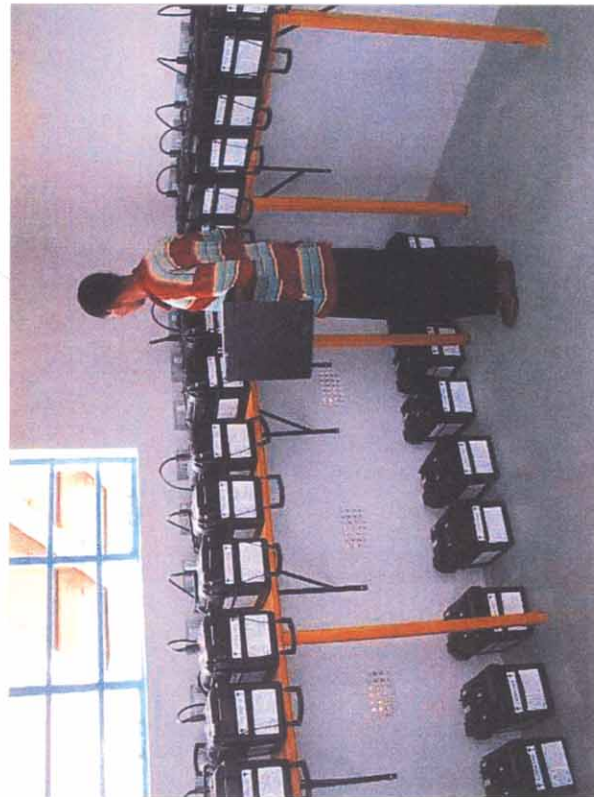
Indoor view of Battery Charging Station
