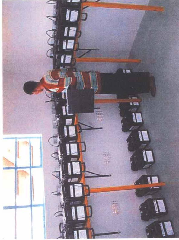
Battery Charging Station 屋内
