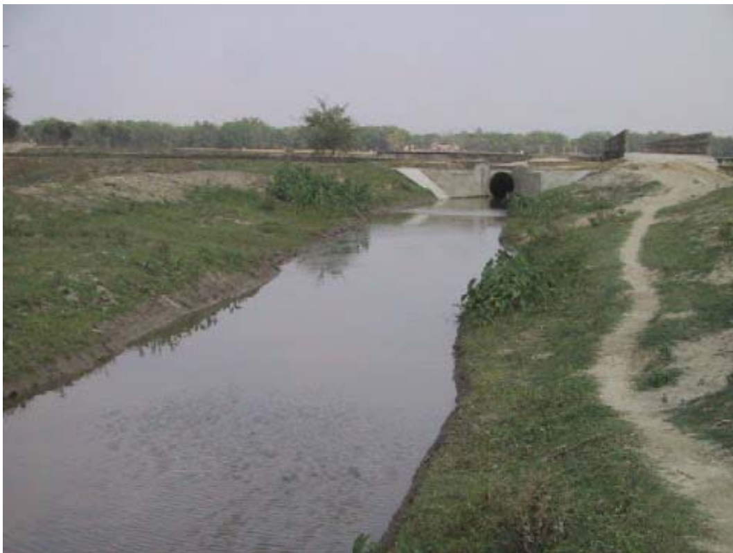
Suksena Canal at the location of siphon crossing the Sunsari River. The irrigation water usually reaches up to this point and irrigate the nearby areas along the canal though it is not enough.
