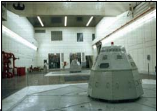
KL-I P/S (Underground)
