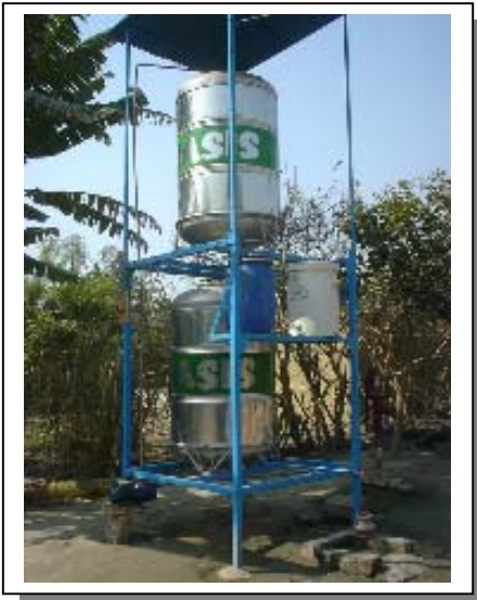
Site for activated alumina unit Near tube well no.108 Before installation (upper) Newly drilled tube well and installed unit (left).
