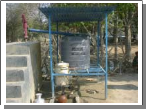
Site for passive sedimentation unit (PS3) Tube well no.155 Before installation (upper) Installed unit and initial experimental operation (right).
