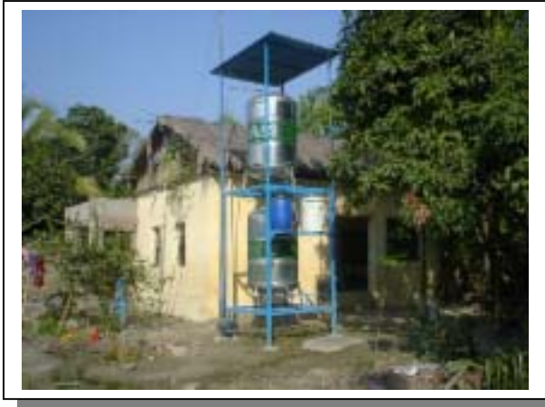
Before and after installation. Site for activated alumina unit I.D. No. 131 New tube well drilled for experiment.
