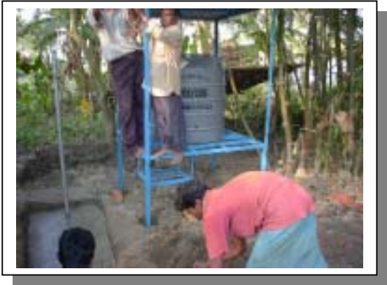
Site for passive sedimentation unit (PS2) East of tube well no.84 Before installation (upper) Installation work of the unit and platform construction (right).
