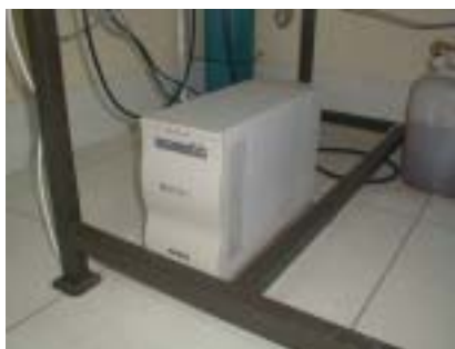
UPS (including stabilizer function)
