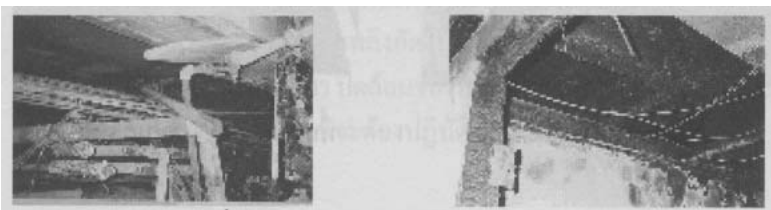
Opening and shaft that are fire spread way
