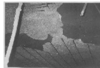
Damaged building floor
