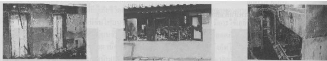
Damaged lift lobby, stair lobby and machine room above stair case
