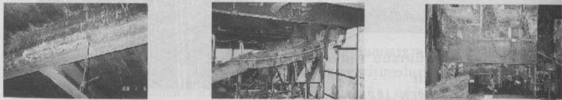
Damaged building structure
