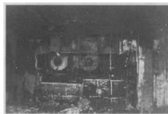
Damaged air handling unit
