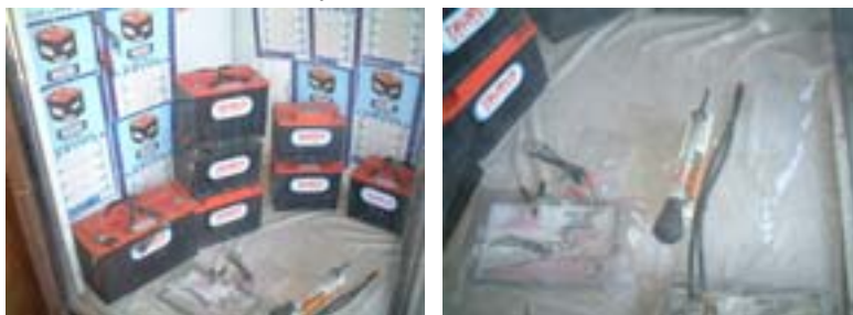
Fig. 7-3-2 (Left) Battery (Right) Battery's tools and parts
