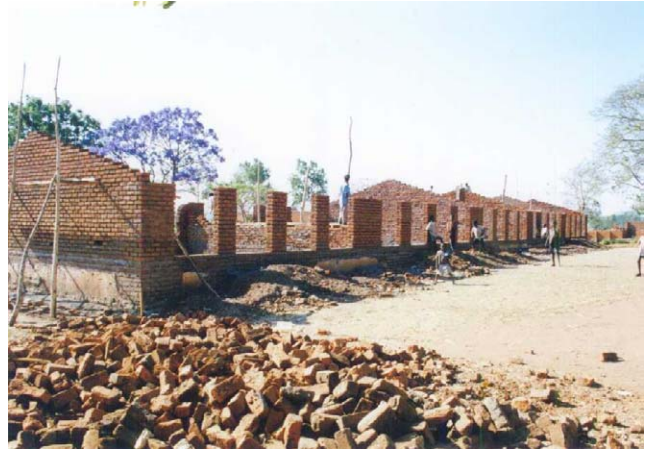
Photo 8-8 School of Under Construction Funded by MASAF (Nambuma TC in Dowa District)
