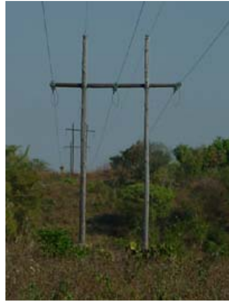
Fig. 3-8-3 66kV Transmission Line
