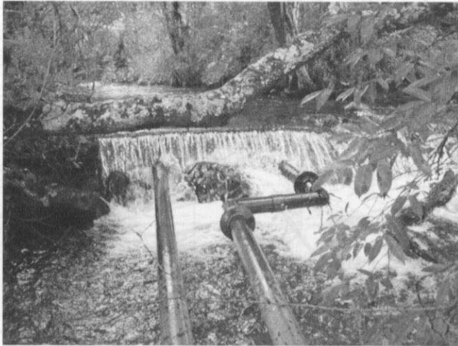
Drinking water facilities installed in Chisenga River
