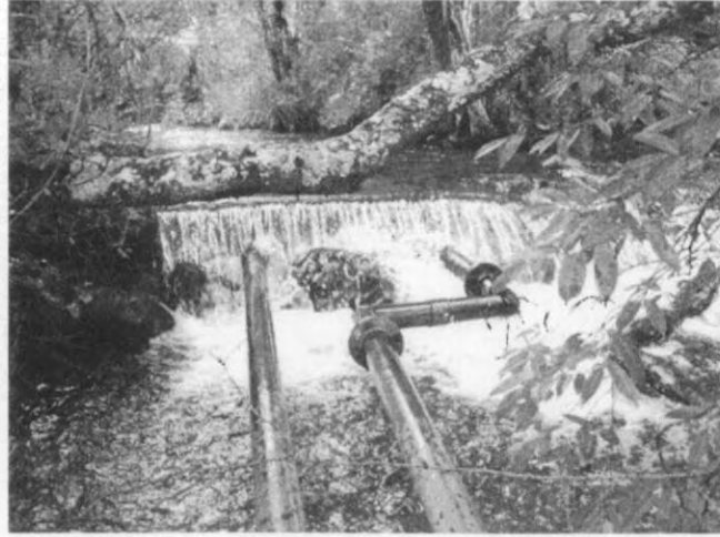
Drinking water facilities installed in Chisenga River
