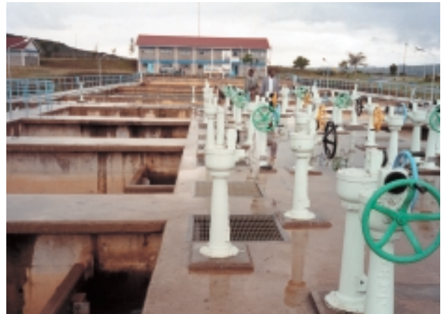
Water purification plant under Greater Nakuru District Water Supply Plan (constructed by Yen-loan)
