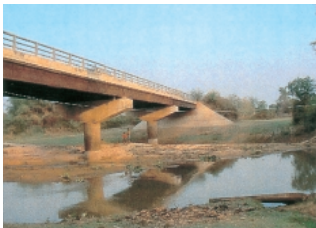
Huai Khum Mum bridge build through the 'Project for Bridge Construction in Northeast Thailand'
