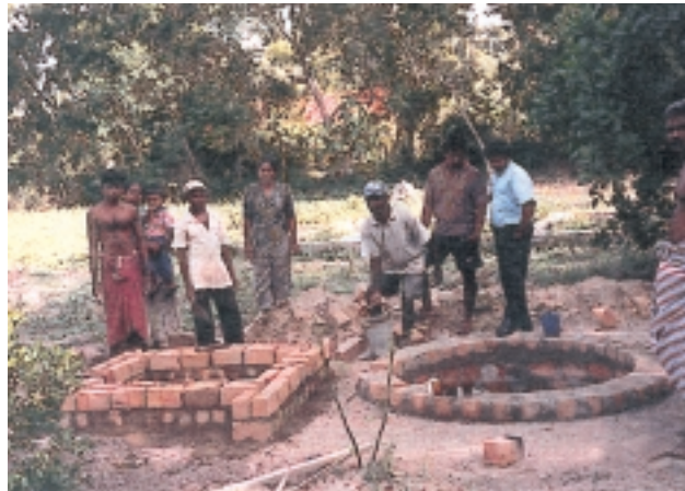
Building of sanitary facilities by local residents ("UC/JICA Joint Study Project on Participatory Rural Development", Sri Lanka)
