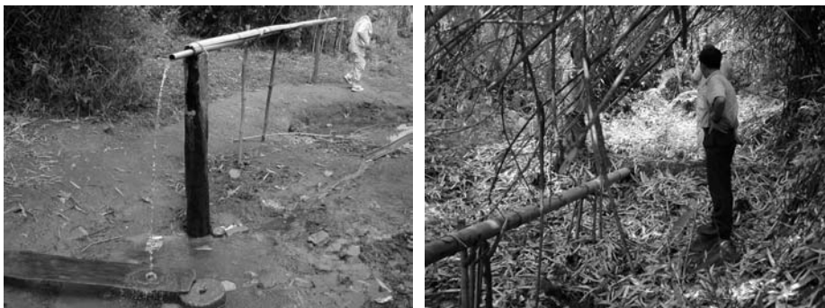
Left: Public piped water supply system is made of bamboo and woods at Dak Ui commune in Kon Tum province. A board and a stone are used for washing cloths. PVC pipe is recently used for reinforcement. Right: Water intake at spring
