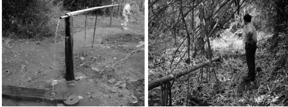
Left: Public piped water supply system is made of bamboo and woods at Dac Ui commune in Kon Tum province. A board and a stone are used for washing cloths. PVC pipe is recently used for reinforcement. Right: Water intake at spring
