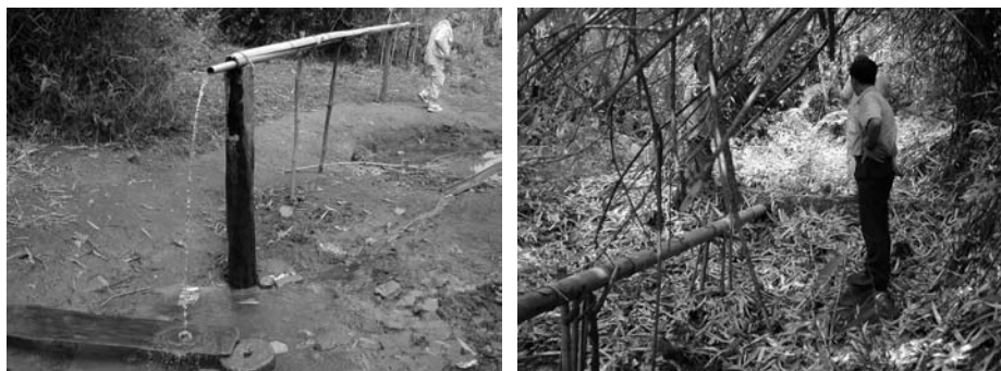
Left: Public piped water supply system is made of bamboo and woods at Dac Ui commune in Kon Tum province. A board and a stone are used for washing cloths. PVC pipe is recently used for reinforcement. Right: Water intake at spring
