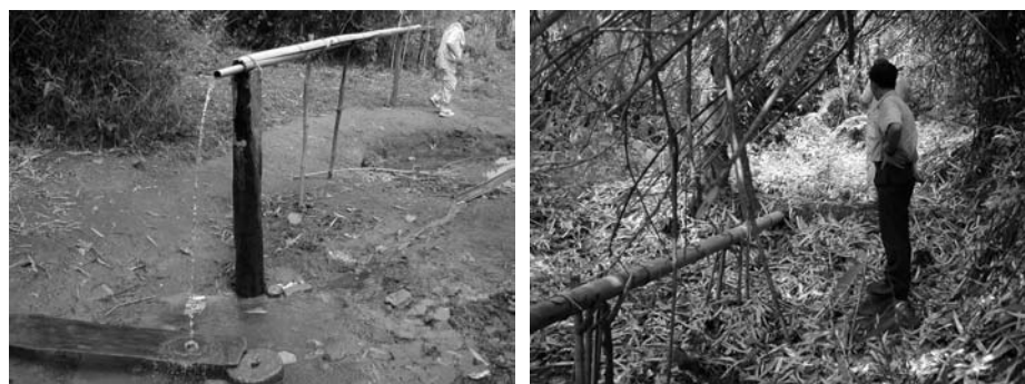
Left: Public piped water supply system is made of bamboo and woods at Dak Ui commune in Kon Tum province. A board and a stone are used for washing cloths. PVC pipe is recently used for reinforcement. Right: Water intake at spring
