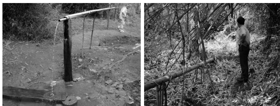
Left: Public piped water supply system is made of bamboo and woods at Dak Ui commune in Kon Tum province. A board and a stone are used for washing cloths. PVC pipe is recently used for reinforcement. Right: Water intake at spring
