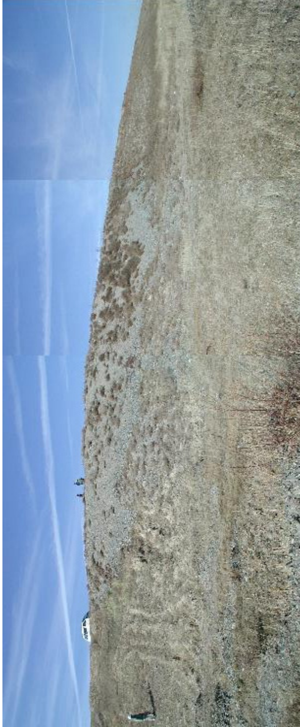
Fig. 6.3-13 Southern Embankment Outside Status of the 3 rd Ash Pond (On October 5, 2001 shooting)
