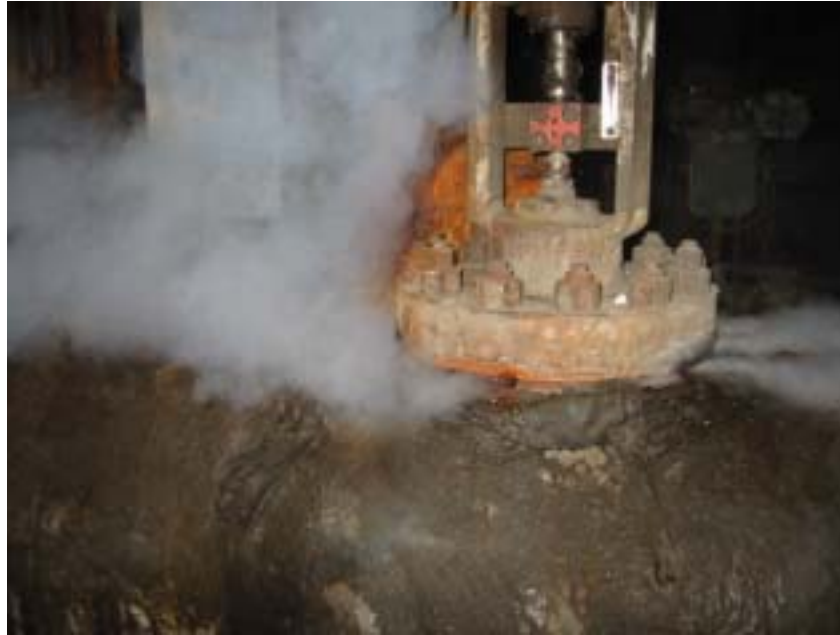
Fig. 5.2-9 The Leakage Situation of the Feed Water Valve
