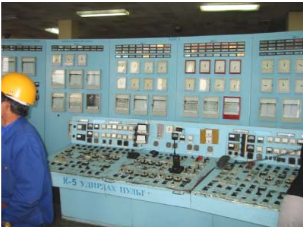
Boiler Control Panel (Existing)
