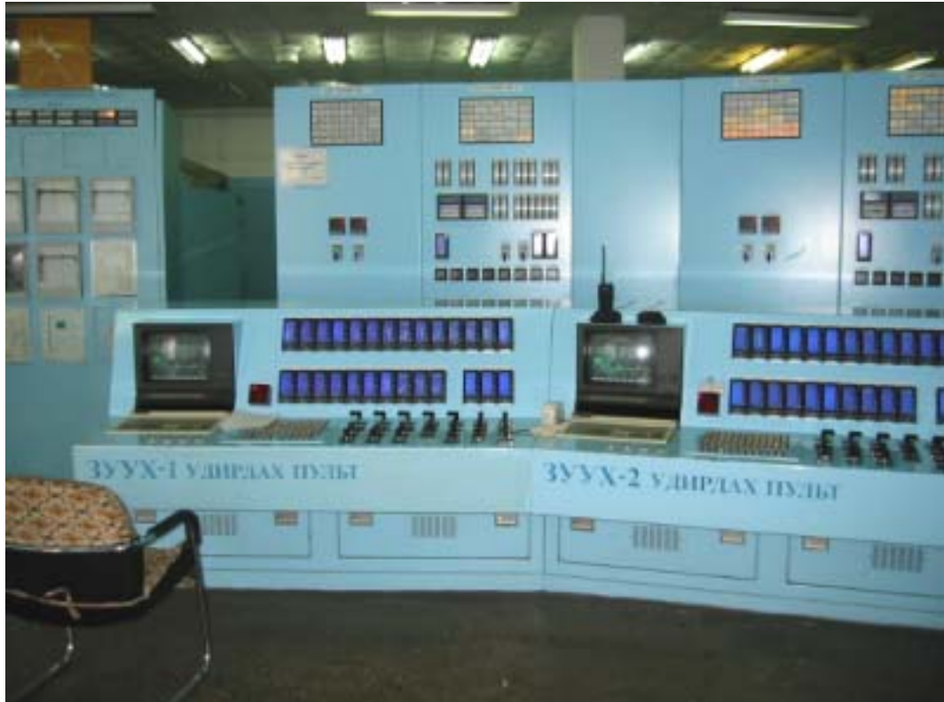
Boiler Control Panel (Rehabilitated)
