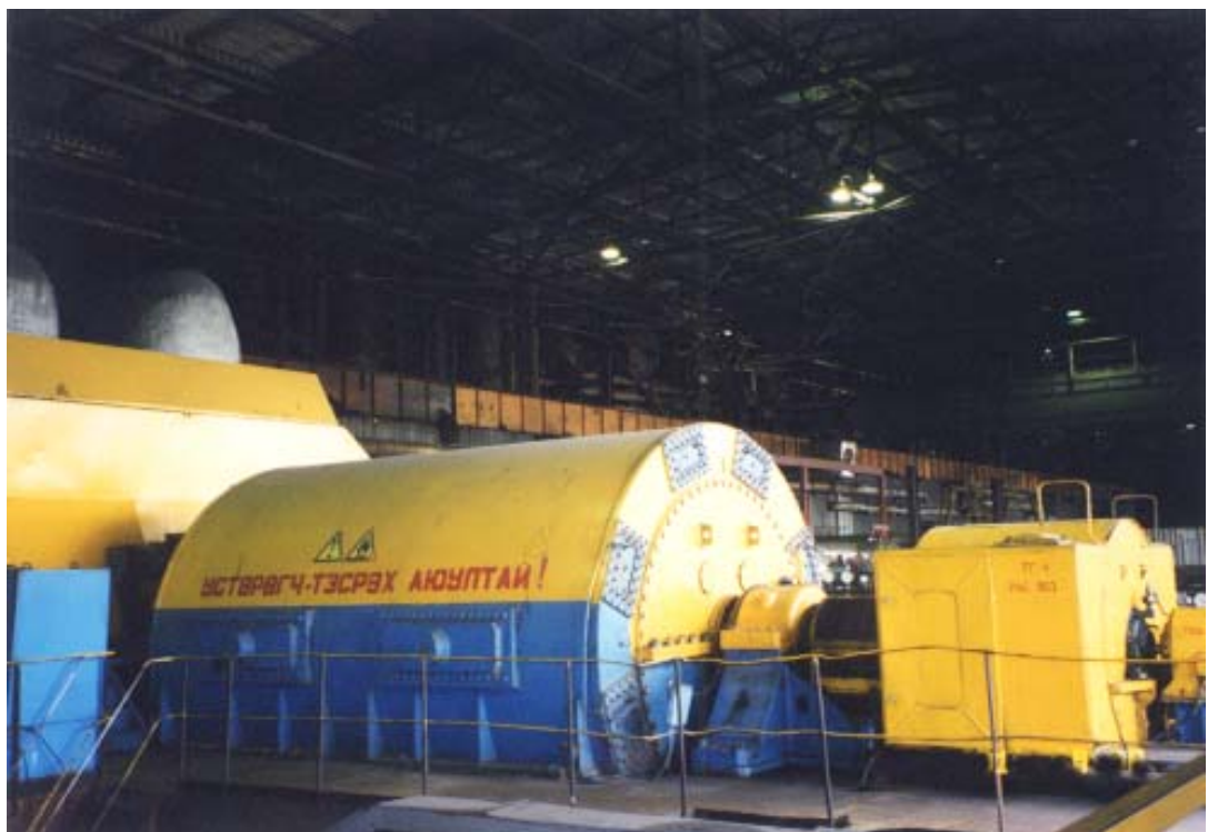
Generator & Exciter (Existing)
