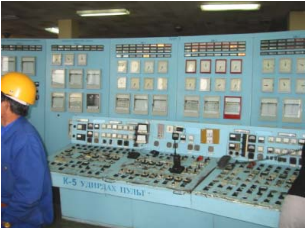
Boiler Control Panel (Existing)
