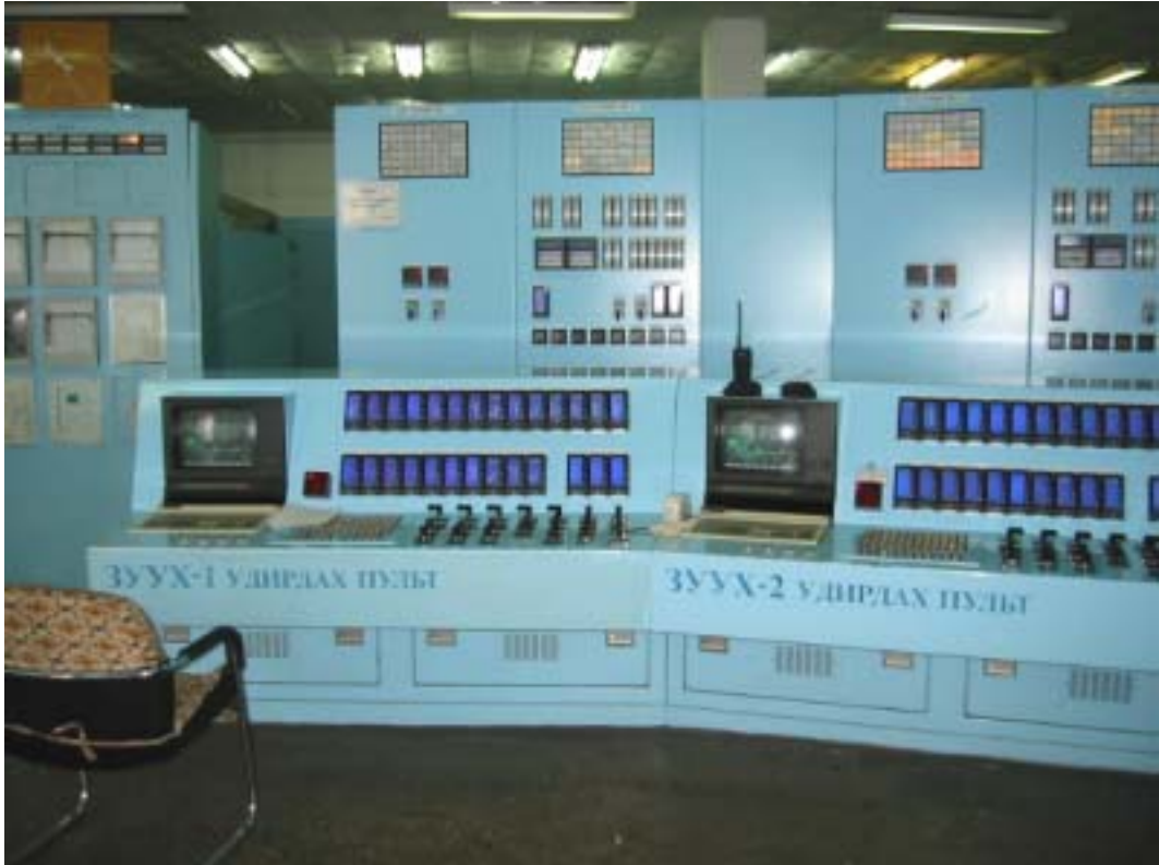
Boiler Control Panel (Rehabilitated)
