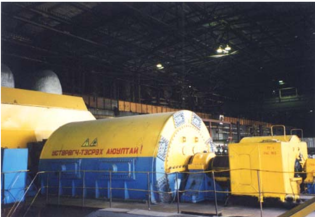
Generator & Exciter (Existing)
