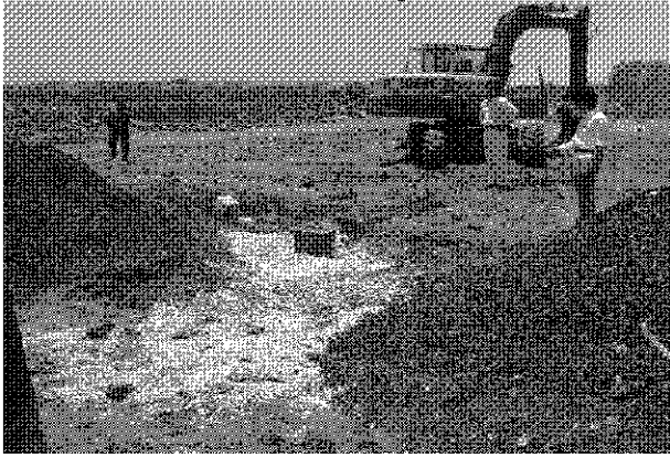
<Groundwater Monitoring Well>
