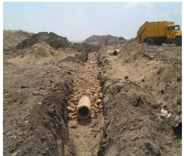
Leachate Collection Pipe
