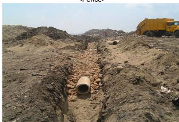
<Leachate Collection Pipe>
