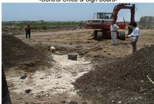
<Groundwater Monitoring Well>
