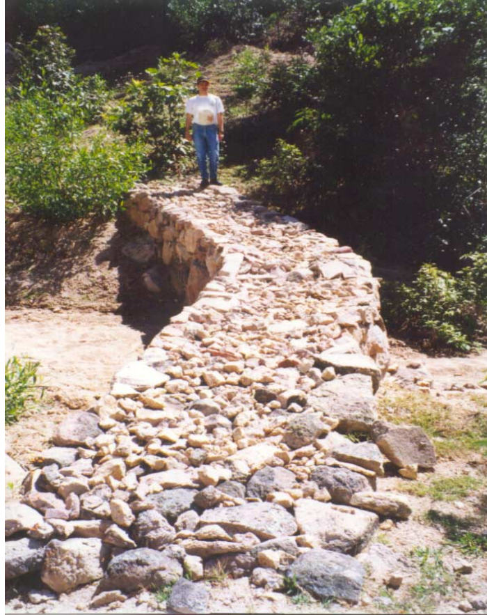
Photo I.5.3 Recently Constructed Dry Masonry Micro-SABO Dam (1993) at the Area of Concepción Dam.
