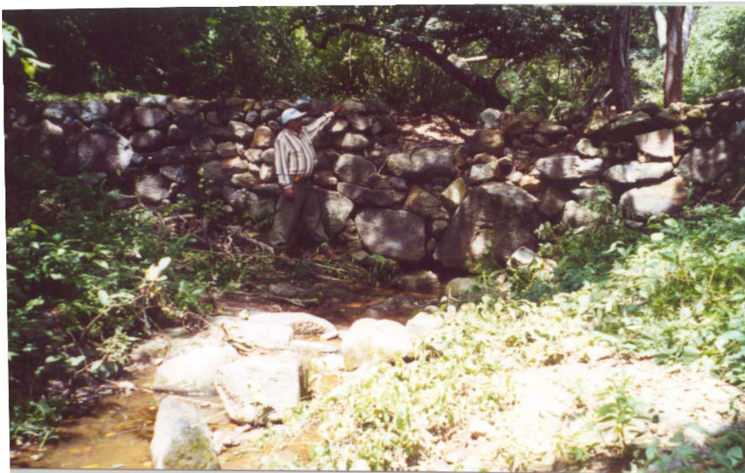
Photo I.5.4 Dry Masonry Micro-SABO Dam Already Filled (H=2m, L=12m) Constructed by SANAA at Concepción Dam Area.
