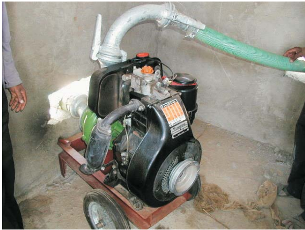
Pump Installed by The Study
