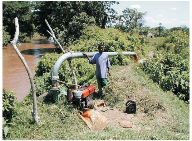
Small Pump Installed by A Private Investor
