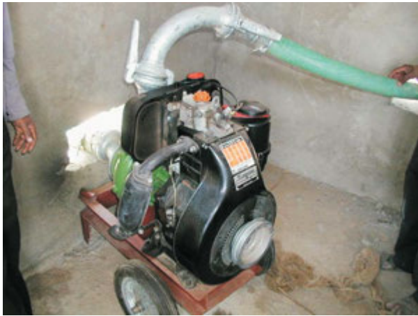
Pump Installed by The Study
