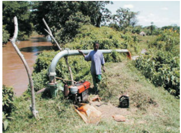
Small Pump Installed by A Private Investor
