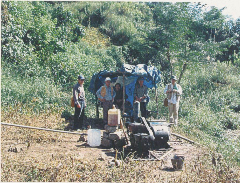
Water pump (Dong Pao river site)
