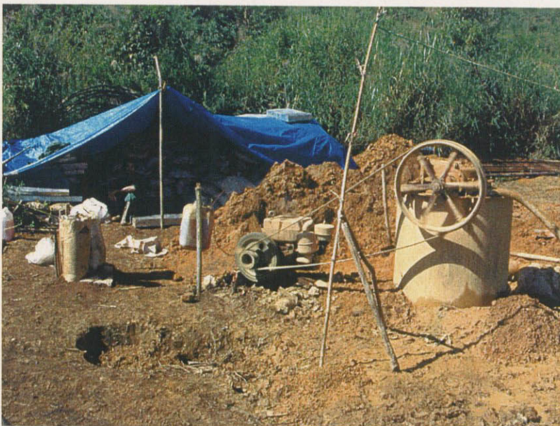
Mixer for drilling mud
