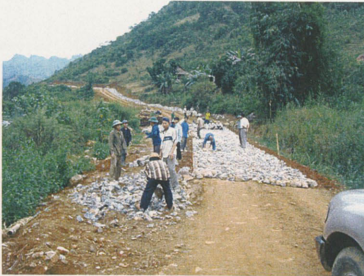
Road construction of main road near Old Dong Pao (Vietnam governmental work)
