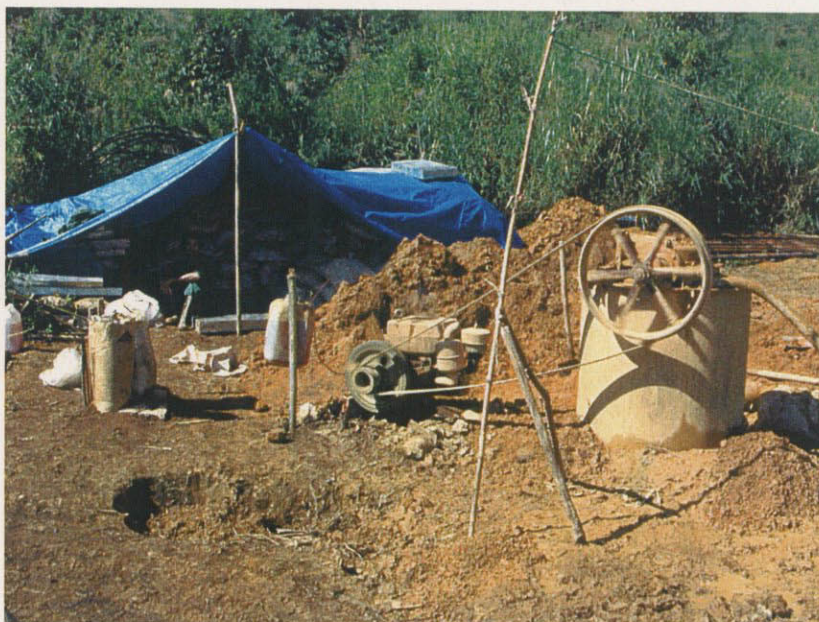
Mixer for drilling mud
