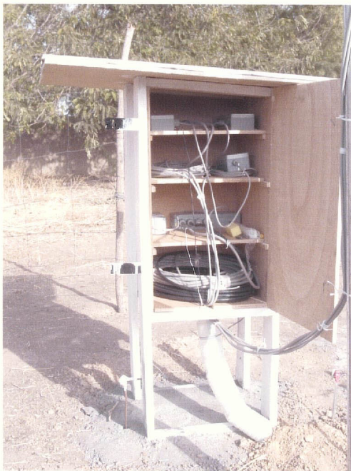
Storages for data measured and batteries
