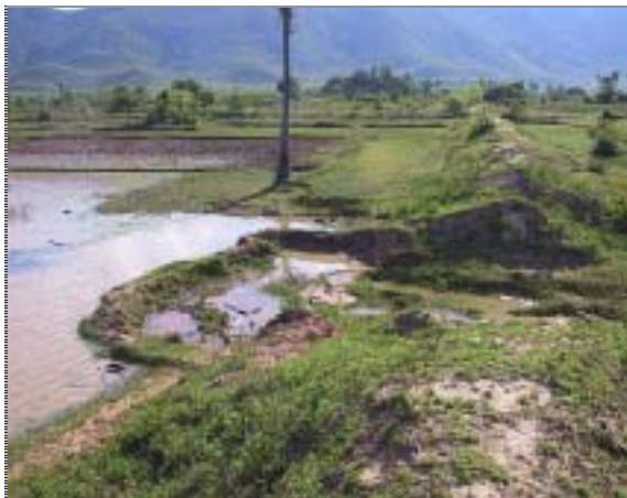
Dike was flushed away for 10 m long
