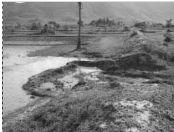
Dike was flushed away for 10 m long
