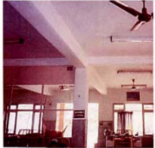
Very thin beam in transverse direction; may cause failure during big earthquake in that direction
