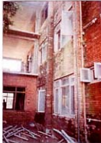
Grass on the wall; cause of deterioration
