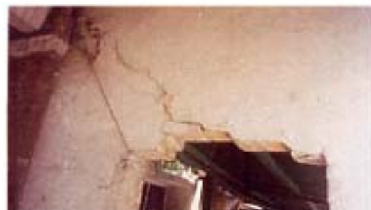
Diagonal cracks from opening
