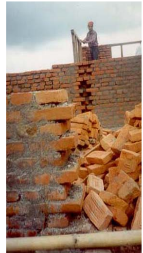
Construction Practice itself makes masonry buildings weaker in corner and joints
