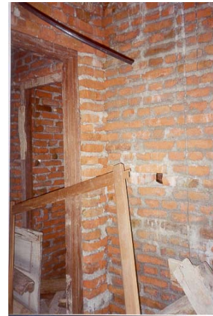
Very poor connection between two orthogonal walls
