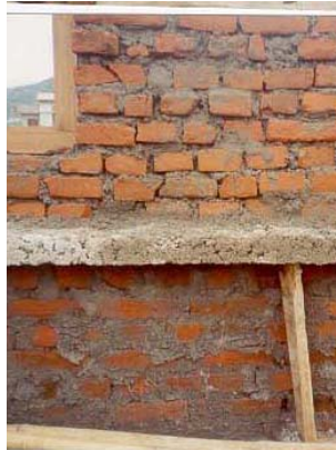
Improper bonds between walling masonry units
