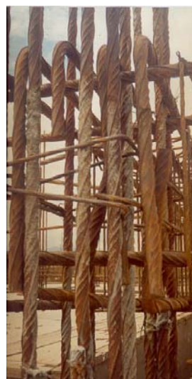
Insufficient beam bars anchorage
