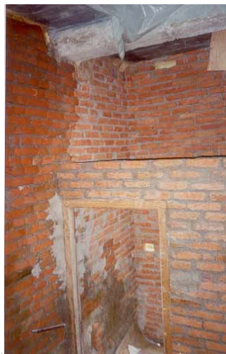
Unsupported 9" wall of about 13' height near staircase
