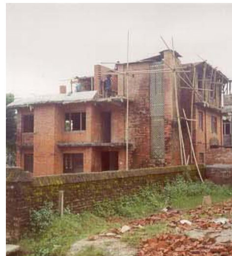
Three story masonry building, the construction practice of erecting two parallel walls first by leaving alternate brick projected out, which make the building weaker can be seen in top floor
