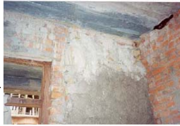
No connection between two walls, one in stone masonry and other in brick masonry
