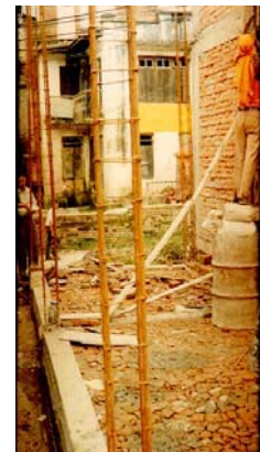
Reinforcement work of column showing 4 number of column bar and large column
