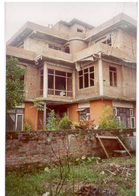
Four story masonry building under construction, Ground floor in mud mortar and remaining floors in cement mortar
