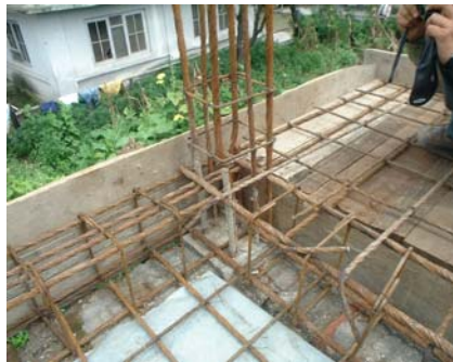
Photo 6.1.7 RC Structure (beam length shortage)
