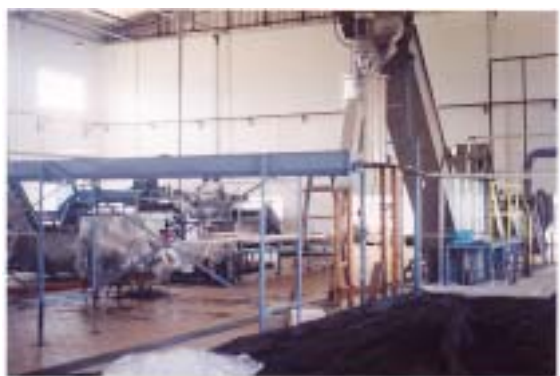
Tropical Fruits Processing Plant in Tome-Açu (Production Line )
