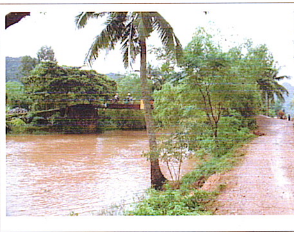
Picture 2: Approach road on right bank, down-stream, and 2.0m wide only
