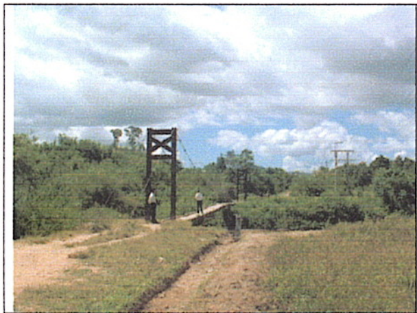
Picture 1: On the alignment of proposed bridge (after demolition of existing one)
