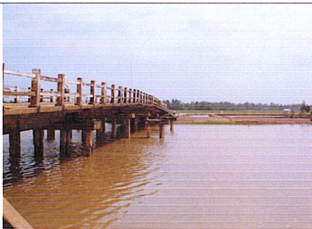
Picture 1: On proposed bridge alignment from right bank, 2 protection pile groups to be removed.
